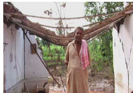
Younas Masih and his damaged house
