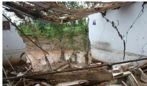
View of a damaged house in Tarnab Farm
